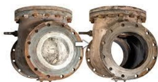
Figure 2: Serious pipe blockages caused by struvite deposits. ©apexengineering
